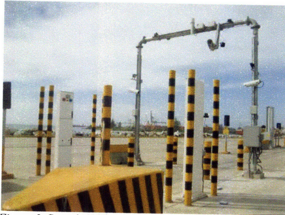
Figure 3. Sample RPM Equipment at SFI location
